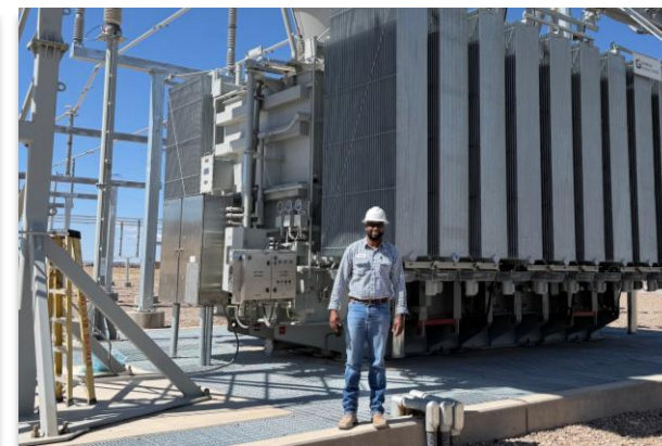
Cape Station power transformer
